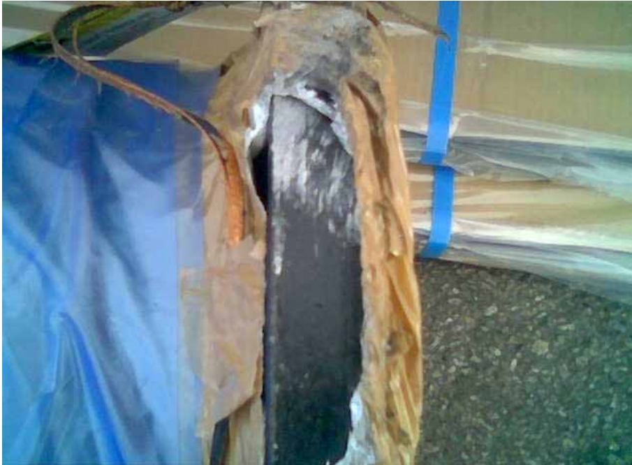
Damage caused to mating surface of fuel hose that could have been avoided with better packaging
